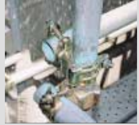
Tightening of step clamp
